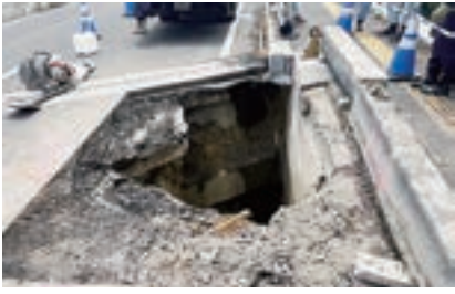
▲新田橋袂の路面陥没
